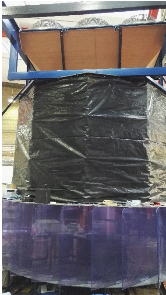
(a) View of the generator
