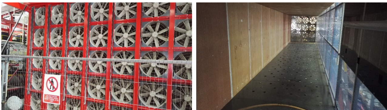
(a) View of the fans
